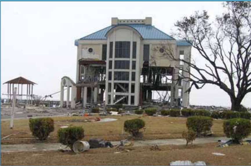
Figure 17. Extensive damage to this building in Biloxi, MS suggests that the storm surge reached as high as 20 feet
