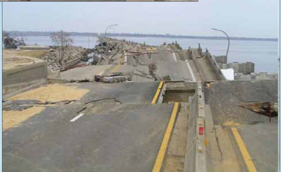
Figure 9. Storm surge damage to Hwy 90 bridge heading east out of Biloxi, MS towards Ocean Springs; in addition to becoming unseated from its piers, the bridge deck was displaced laterally approximately 20 feet
