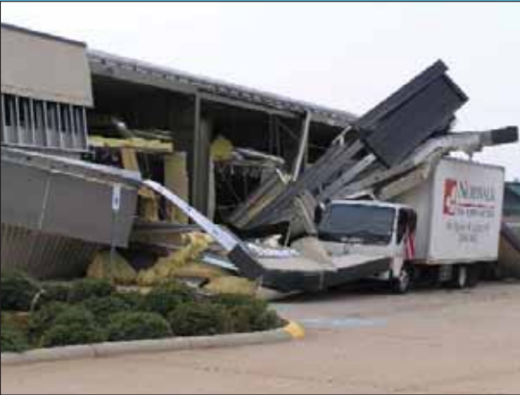
Figure 14. Collapse of the front wall and loading bays of a commercial building in Gulfport, MS
