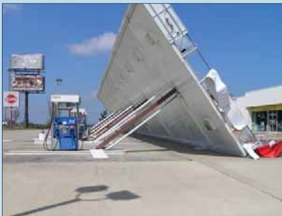
Figure 5. Damage from the force of the wind to the canopy columns at a gas station in Hattiesburg, MS
