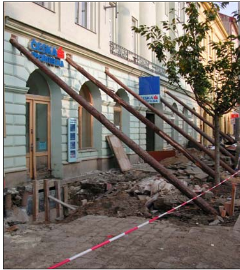
Figure 19. Settling of the pavement soil is evidence that water may have undermined this building. The structure is shored up by temporary supports to prevent collapse
