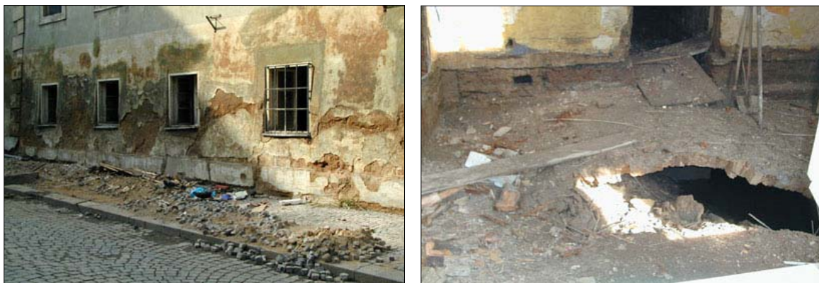
Figure 17. Severe masonry damage on the outside, and floor collapse inside a building in Lesser Town (photos courtesy of Radio Prague)
