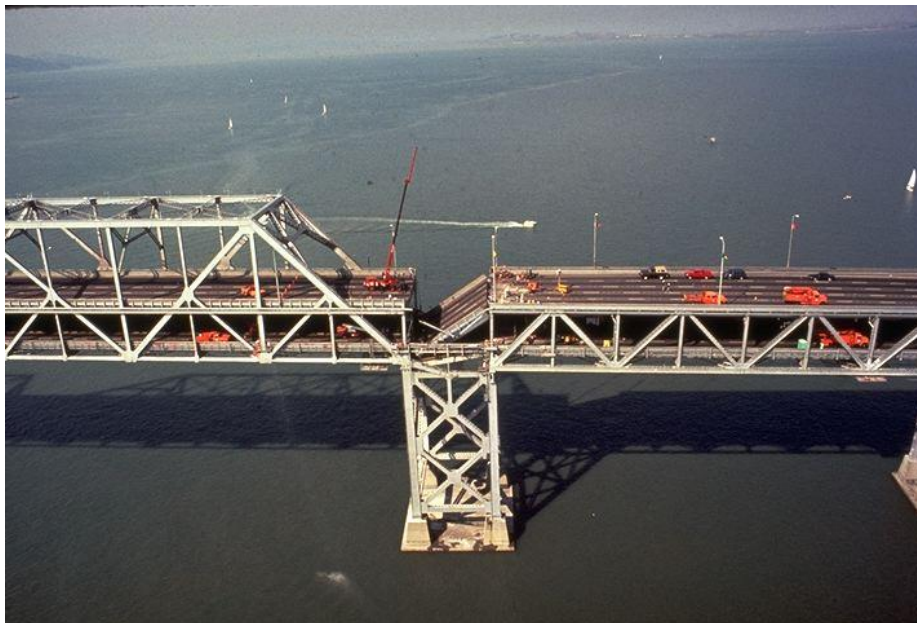
Figure 2: Damage to the San Francisco-Oakland Bay Bridge, spanning the San Francisco Bay, as a result of the 1989 Loma Prieta Earthquake; a seismic retrofit of the bridge is ongoing in 2009
