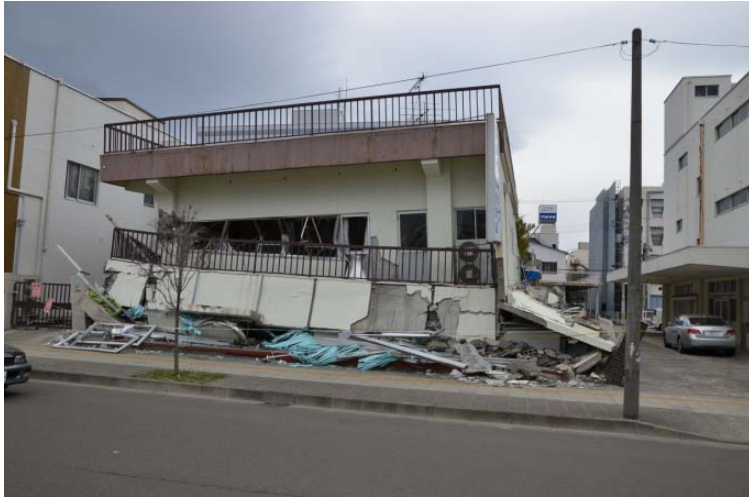
Figure 2: Collapsed building due to ground shaking in Sendai in Miyagi Prefecture (Source: RMS reconnaissance)
