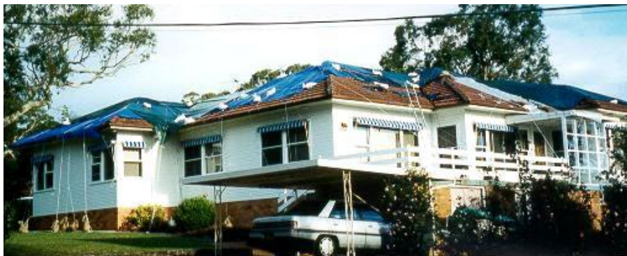
Figure 8: Tarpaulins covering the roof of a residential structure in the eastern suburbs of Sydney following the 1999 Sydney Hailstorm (Source: http://willoughby.ses.nsw.gov.au/Hail.html )
