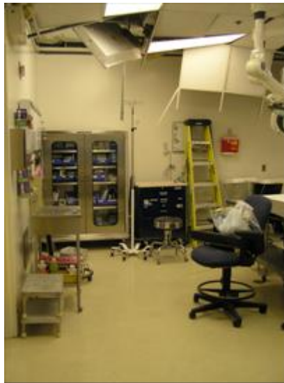
Figure 15: Non-structural damage to equipment and ceiling grids at Kona Community Hospital
