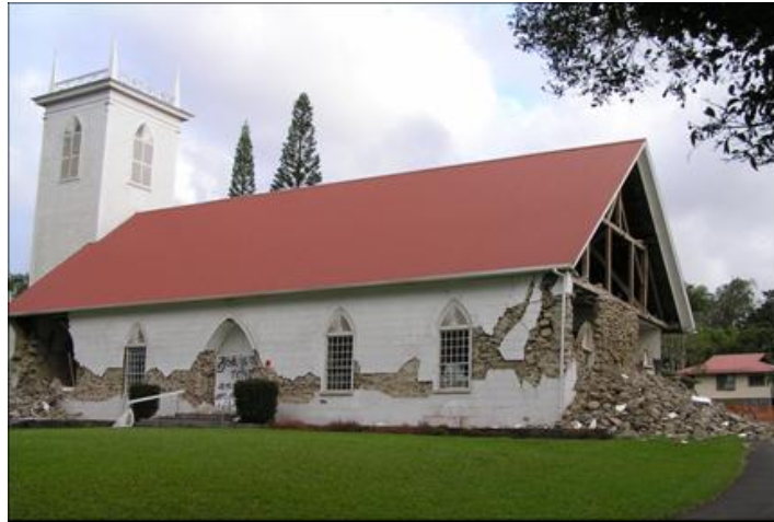
Figure 13: Severe damage experienced at Kalahikiola Church in Kapaau
